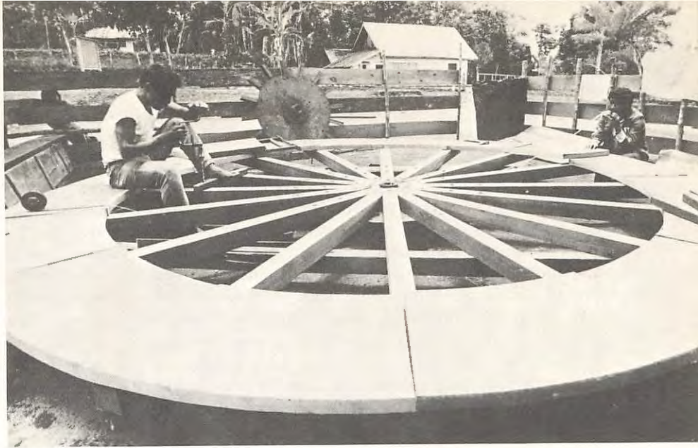
Villagers construct a water wheel assisted by a KKN student from Syiah Kuala University, Aceh.
