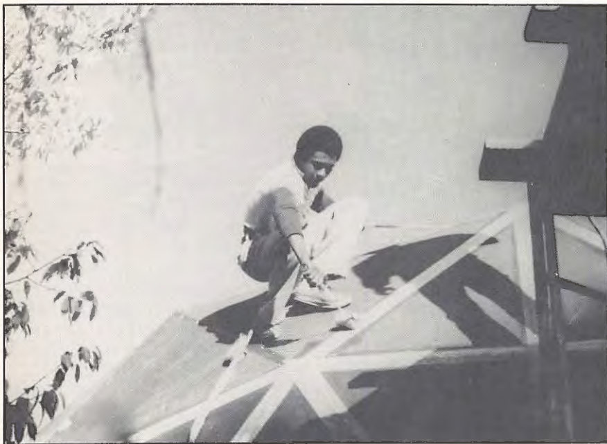
Taping the seams at the top of the dome, a student holds onto a rope for support.
