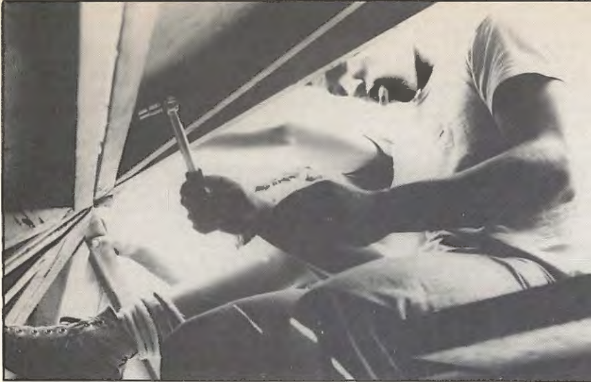
In the last phase of dome construction, a student bolts panels into place.
