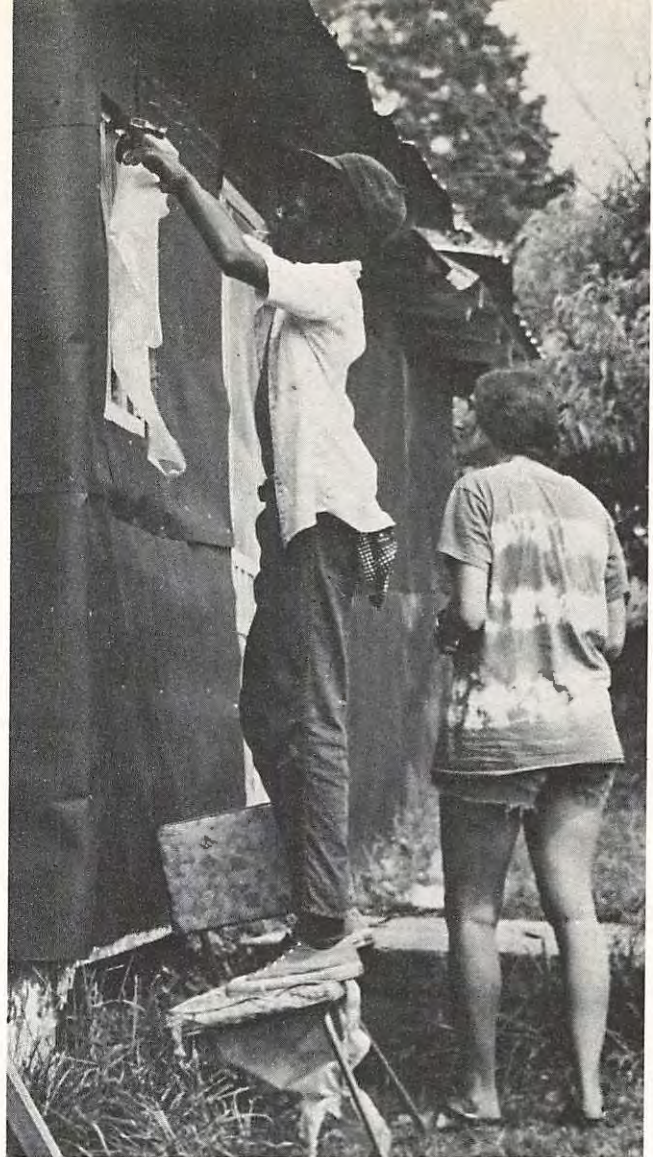
A Neighborhood Youth Corps member joins CHIP workers on a room-addition project for a Charlottesville area resident.
