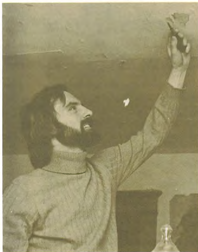
John Gross, a U. of Mass. public health student, chips lead-based paint off a ceiling in a house near the Amherst campus.
