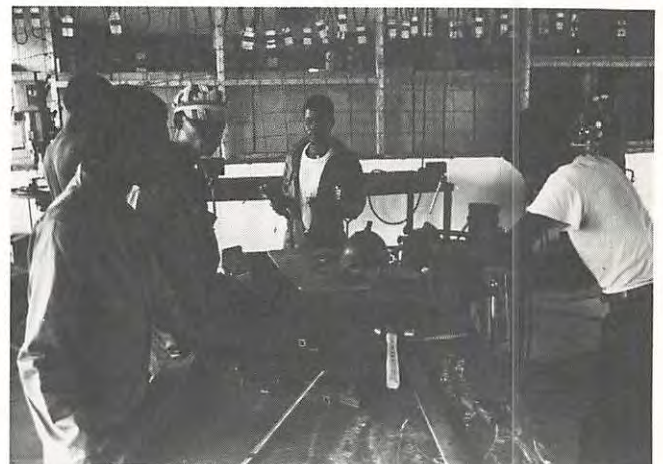
A welders brigade in Mahalapye in east Botswana at work on a project.
