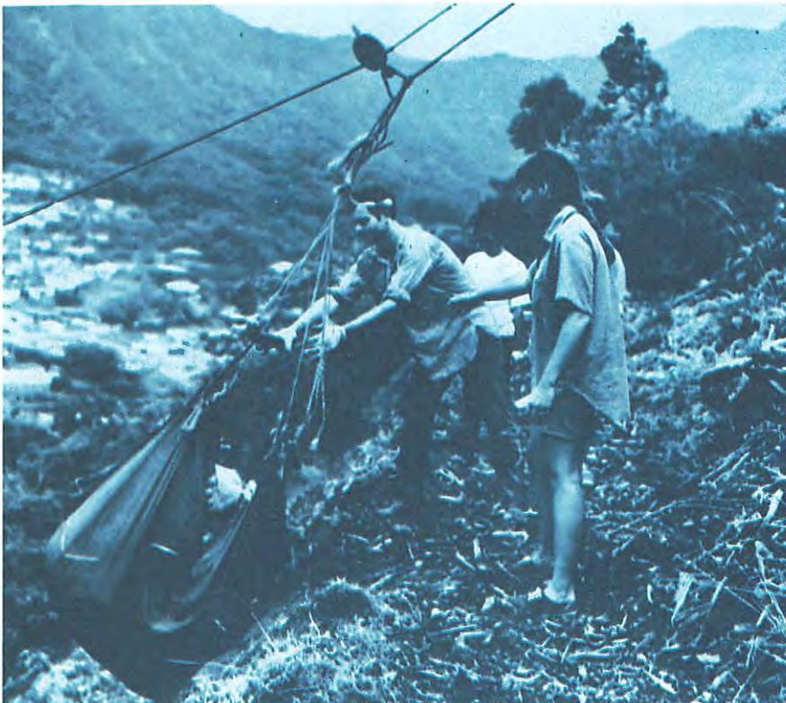
Unloading fertilizer from a cable lift in "Pao's Cut," University of Hawaii students work to make a Manoa Valley hillside green again. The job took a year to complete.
